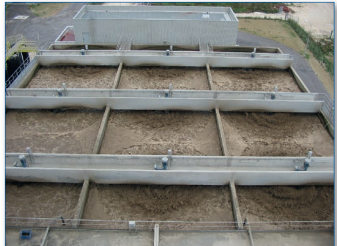
LANDY surface aerator at rectangular basin
