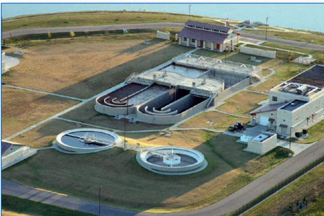
Activated sludge process with LANDY surface aerators
