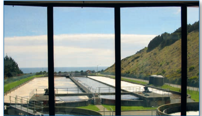
LANDOX flow boosters at WWTP Porirua, New Zealand
