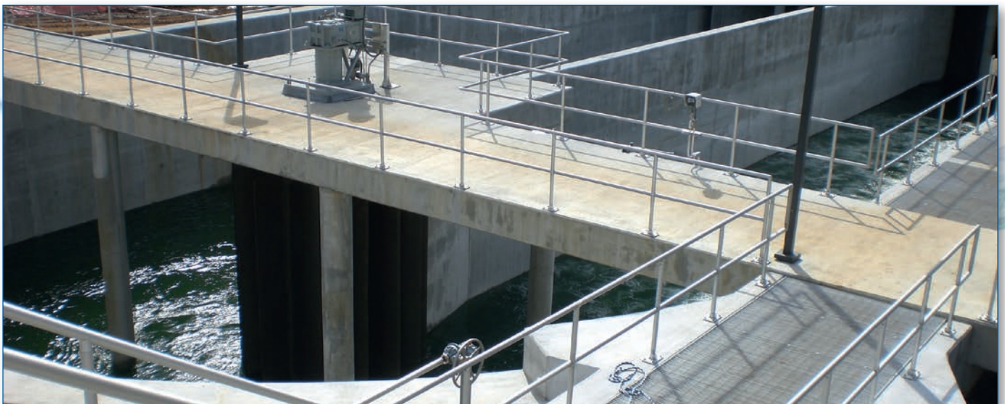
Oxidation ditch with fine bubble diffusers and LANDOX flow booster
